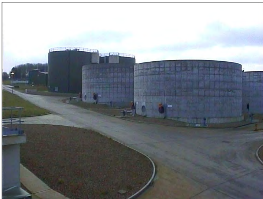
Figure 6 Anaerobic digestion - 2 primary mesophilic digesters (above) and 4 secondaries below
